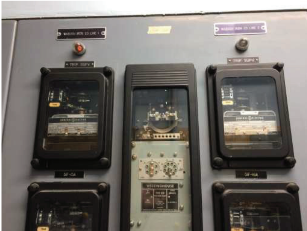
Figure 1: Existing Line Protection Relays (Wabush Terminal Station)
